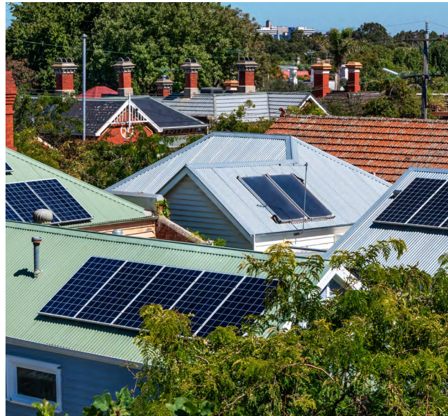
Rooftop solar in Melbourne, Australia.
